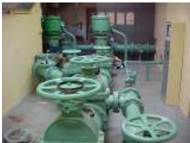
Booster Station, Taos, NM
