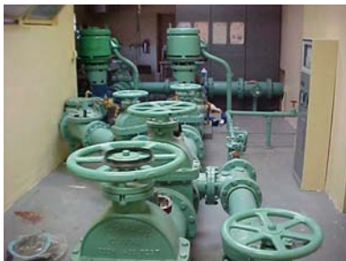
Booster Station, Taos, NM
